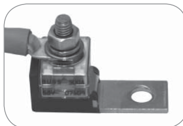
Fig. 7. Fuse MRBF and Positive cable fixed to the CFBAR
